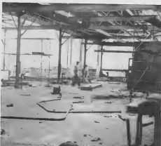
In a scene reminiscent of the Korean War, two workmen dismantle the old welding shop (12). The structure of this building, plus the old carpenter and pipe shops will go to make a 10,500 sq. ft. warehouse space (16). Air conditioned storage will also be added.
